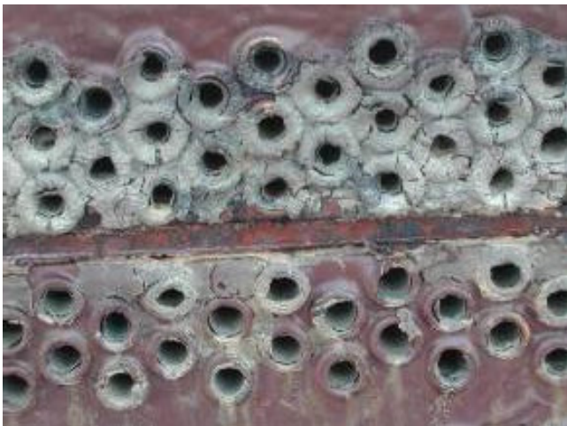
Fig1: Clogged H 2 S Cooler: mud and scale.
