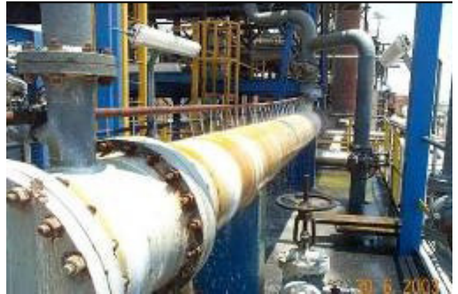
Fig.2: External cooling for the H 2 S Cooler
