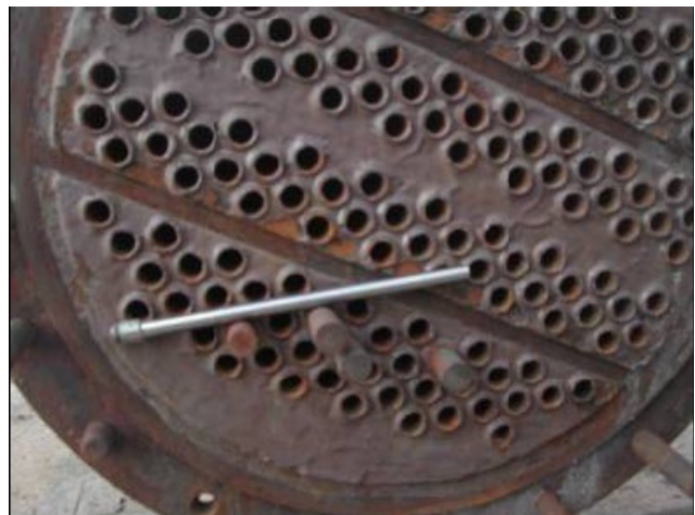
Fig.3: Clean H 2 S Cooler by CQM's ATCS
